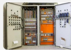
Electrical Cabinet Environmental Monitoring
